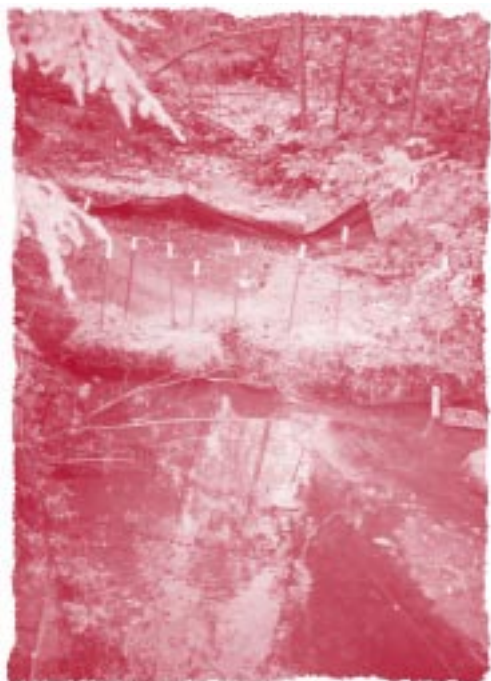
These straw bales in the creek and the collapsed silt fence are examples of inadequate erosion control.
