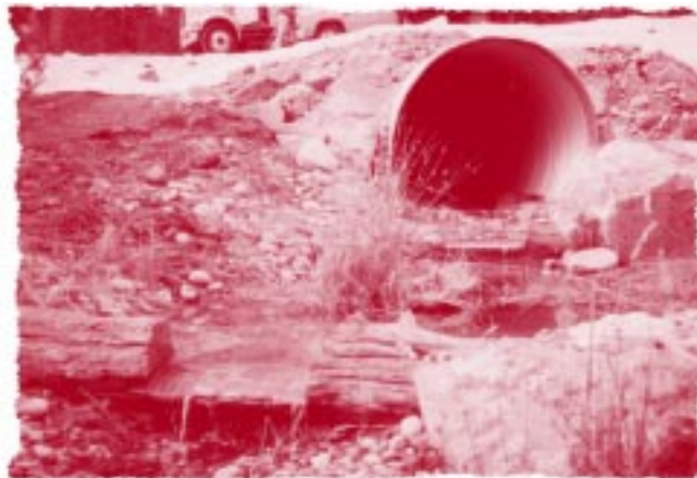
This new culvert in Stables Creek replaced a culvert that prevented fish migration. The new culvert is at stream level and is filled with gravel to simulate a streambed.
