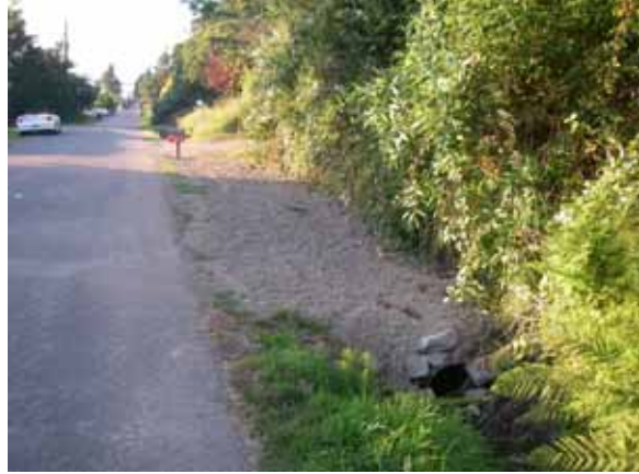
98 th Ave NW After Maintenance: Ditch was excavated, buried culvert was replaced, and catch basin was installed
