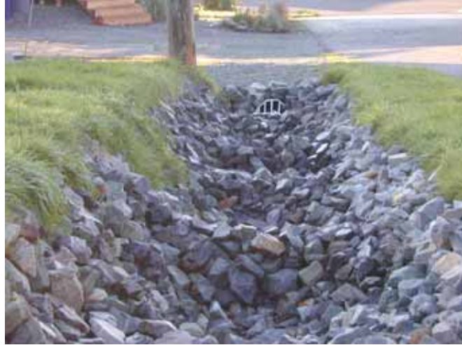
Project WB-M3-03 - Channel improvements and pipe inlet installed by the County in 2004 along 192 nd Street NW
