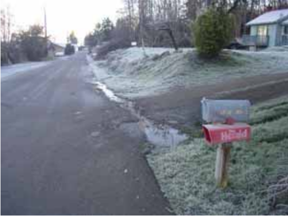
98 th Ave NW Before Maintenance: Surface water flowing around buried culvert and downstream section of filled ditch
