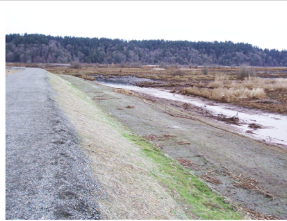
A section of new dike constructed for the Nisqually Delta Restoration Project south of Seattle. The dike features a gravel dike-top road, graduated slope and beaching area. This view is to the waterward side of the new dike showing the early stages of new tidal marsh formation.
