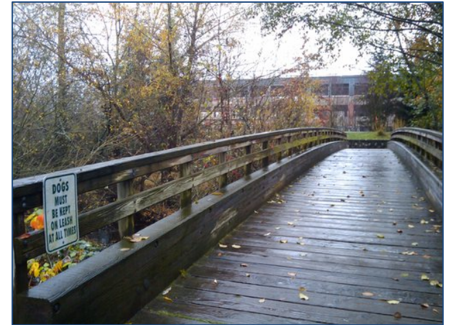
Bridge crossing North Creek Trail in the Schnitzer Development Area in Bothell
