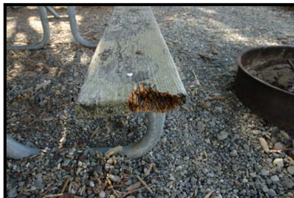
Figure 5: Deteriorating picnic bench at Kayak Point.
