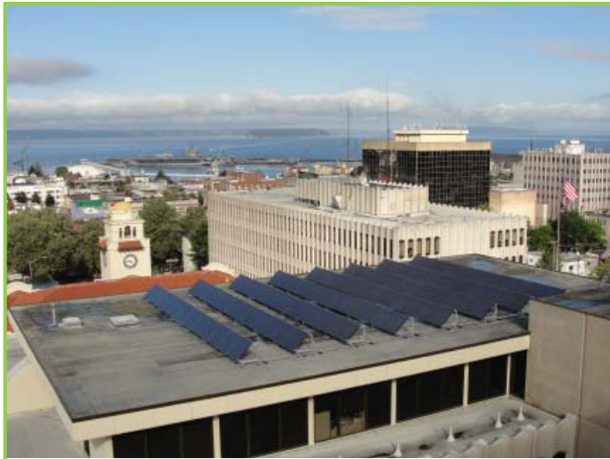
A 16.4 kW solar panel system was recently installed on the roof of the County campus administration building. This solar array will generate electricity for approximately 16 electric vehicle charging stations in the County parking garage and will prevent approximately 21,000 pounds of CO2 from entering the atmosphere each year.
