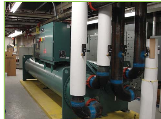
Two new energy efficient water-cooled chillers were recently installed in the the County Campus. These two chillers will save approximately $11,500 per year in energy costs.
